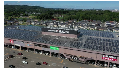
Solar power system installed at the Home Center Musashi store in Natori
