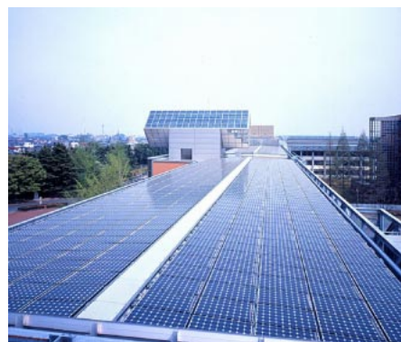
写真1 設置事例(切妻屋根一体型) Photo 1 An application of roof integrated PV module type.
