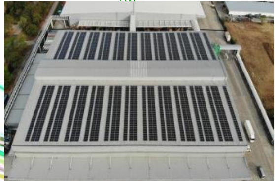
■ New solar rooftop system at Warehouse-2 ; 817.02 kW
