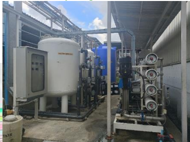
■ SATL Recycling Water Plant
