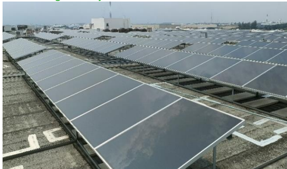
■ Existing solar system 124 kW
