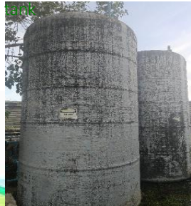
■ Greywater storage tank
