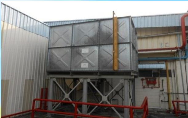
Rain Water Tank
